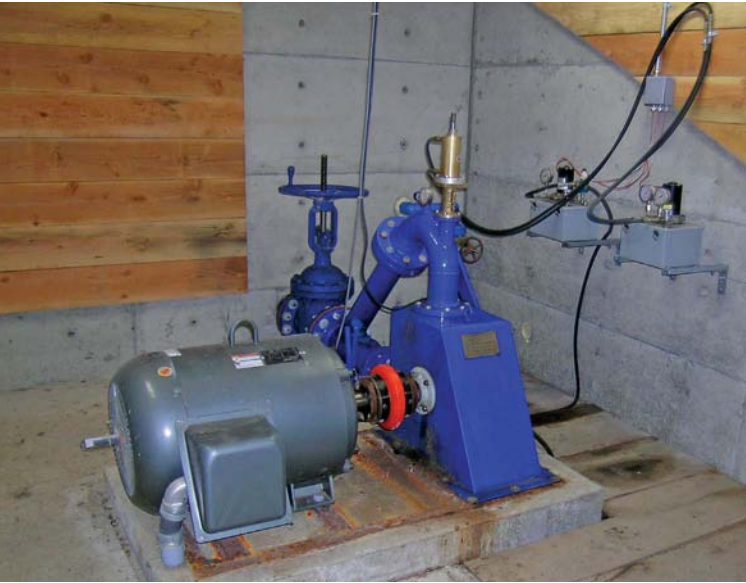
The Canyon Industries turbine consists of a 10.5-inch Pelton turbine and a 60 kW, 480 VAC, three-phase alternator.
