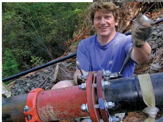
Right: One thousand lineal feet of steel pipe was used in the bottom of the lower penstock. The steep terrain necessitated creative installation and anchoring systems.
