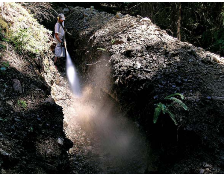
Water pressure was used to blast the trench for the lower penstock.
