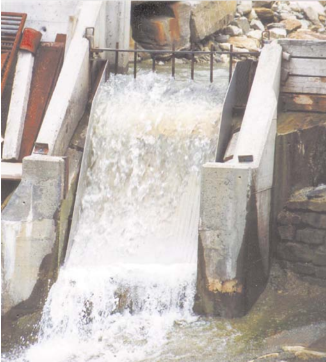
The 4 KW system in Wales after several months without any cleaning, with no detrimental leaf build-up.
