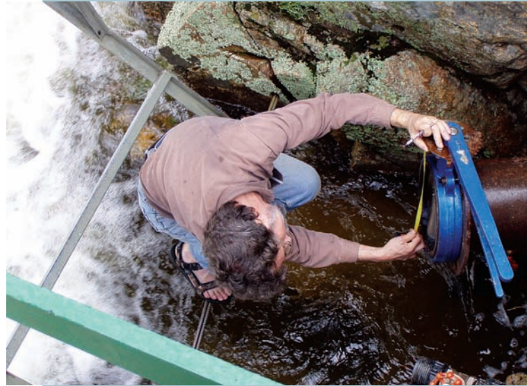
Microhydro turbine manufacturer Paul Cunningham measures the penstock.
