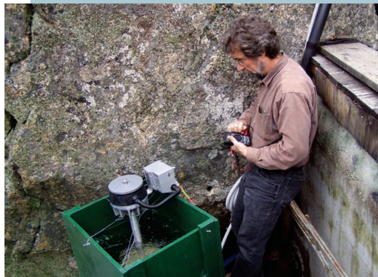
Up and running—the first power output test.
