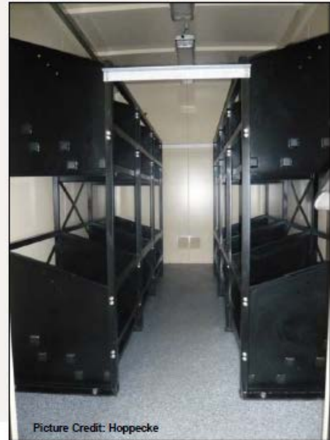
Battery Container (Example)
