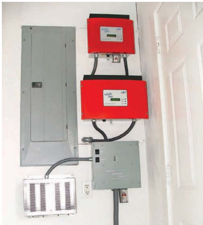
Balance of systems equipment—(clockwise from top right) Sunny Boy 700U inverter, Windy Boy 1800U inverter, Abundant Renewable Energy wind controller, diversion load, and AC mains panel.
