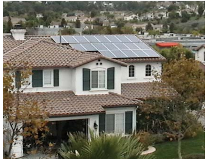
Installed by Palomar Solar in San Diego, CA
