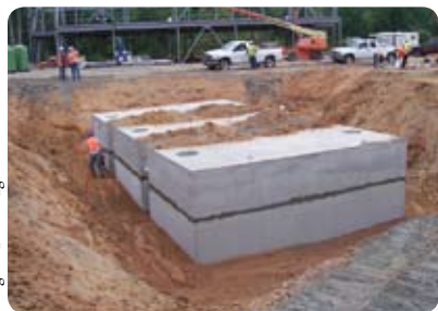
Cistern to store 60,000 gallons of rainwater for irrigation and toilet flushing at a new school being built by the Eastern Band of the Cherokee Indians
